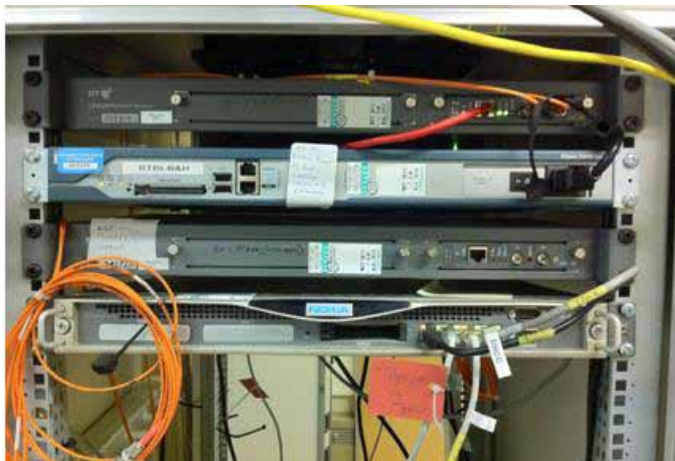
Tracing Cables: Establishing exactly how the existing infrastructure was configured turned out to be one of the biggest challenges for the project.
